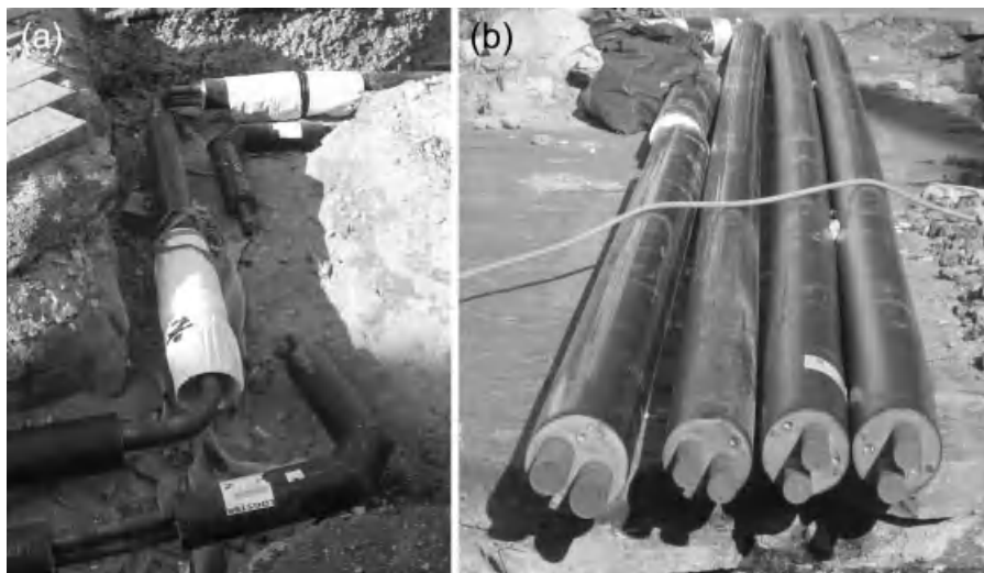
Figure 14.9 (a) Exposed! – part of Stockholm’s district cooling scheme, showing (b) the insulated, two channel pipes used in the distribution net. Photos by D. Banks.
