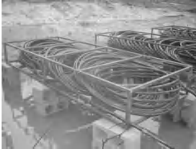
Figure 12.6 Close-up of one of the 'pond mats' in Figure 12.5, each comprising around 200m of coiled HDPE pipes fastened to a steel frame and anchored with concrete blocks. Note the loose bundling of the pipe to reduce thermal interference. Photo reproduced by kind permission of Geowarmth Heat Pumps Ltd.
