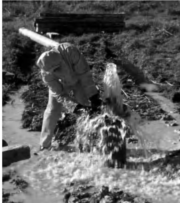
Figure 16.4 An artesian borehole at High Wycombe, UK. Even when steel casing has been securely installed in an artesian borehole, stemming the flow can be a nightmare! Photo by David Banks.
